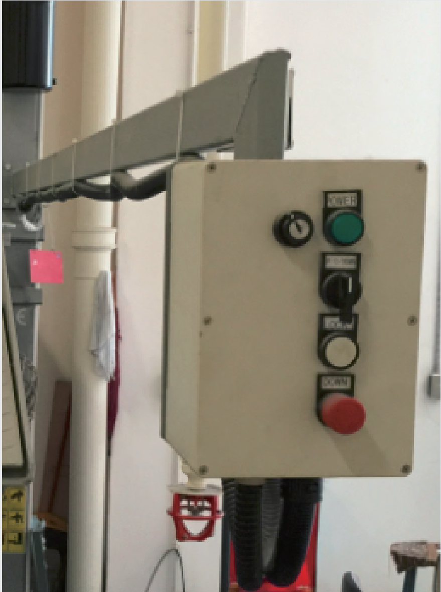
Operation and control system both in one box, cannot secure the operator from electric shock
